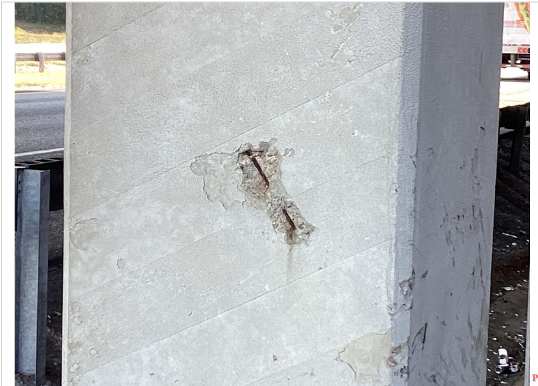
Bent1 = Column B left - popouts
