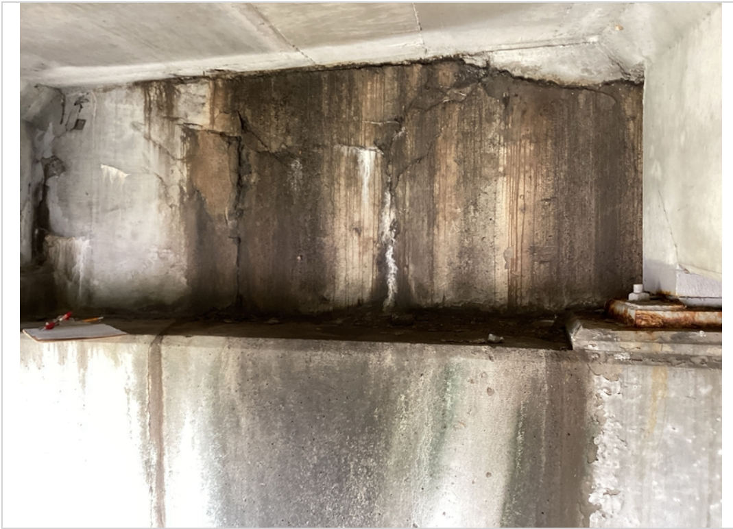
Abutment 1 back wall between beams K & L - Hairline cracks with leaching
