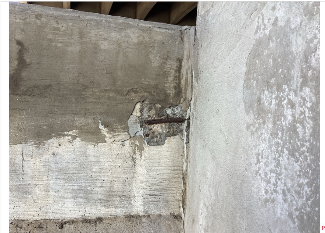
I - 75 East - U.P. Bridge rail in front of columns F & G - popouts
