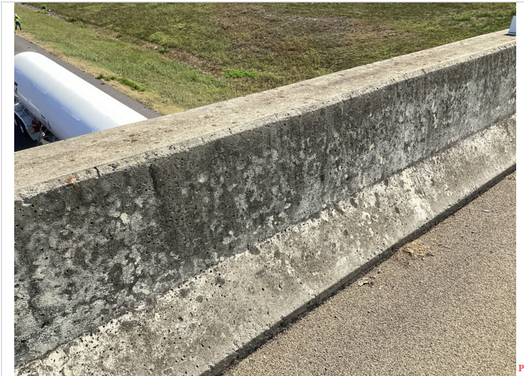
Deck 3 left rail - hairline cracks, aggregate voids (typical all)
