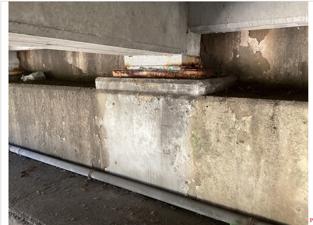
Bearing C abutment 2 - Moderate corrosion (Typical other bearings both abutments)
