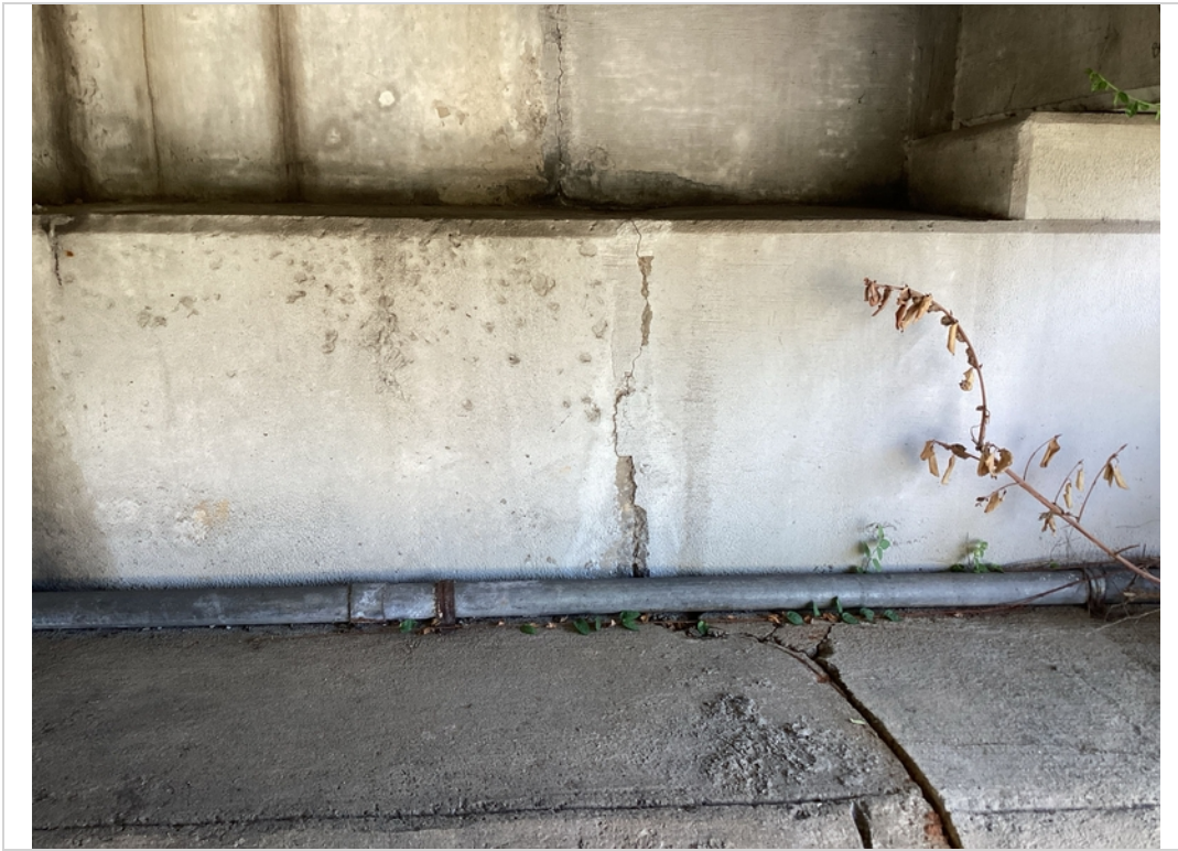
Abutment 2 cap between beams K & L - Cracking up to 1/16"
