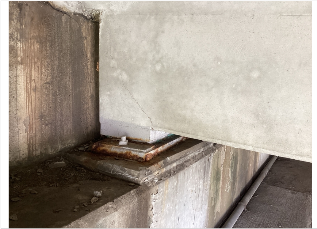
Span 1 Beam K right at abutment 1 - Diagonal hairline crack
