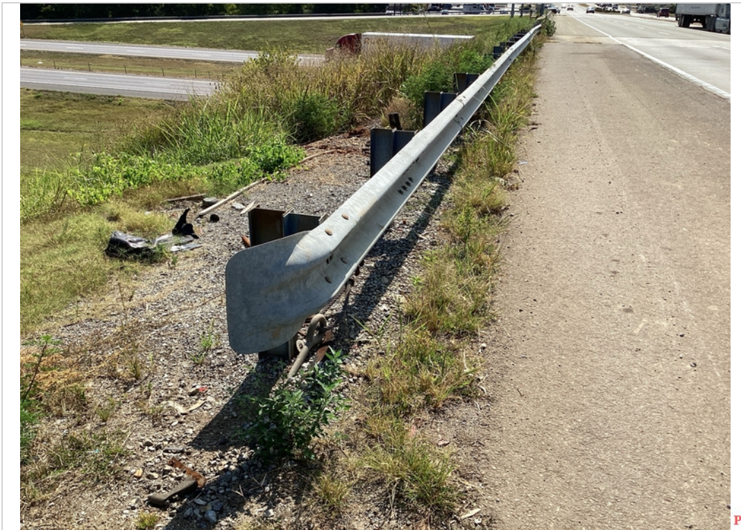
Approach 1 left rail terminal- substandard
