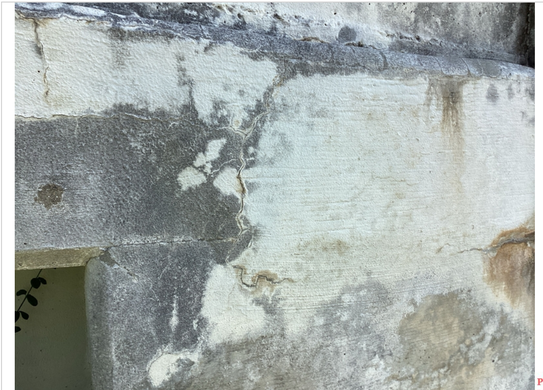
Wing 2 right - Hairline cracks with leaching
