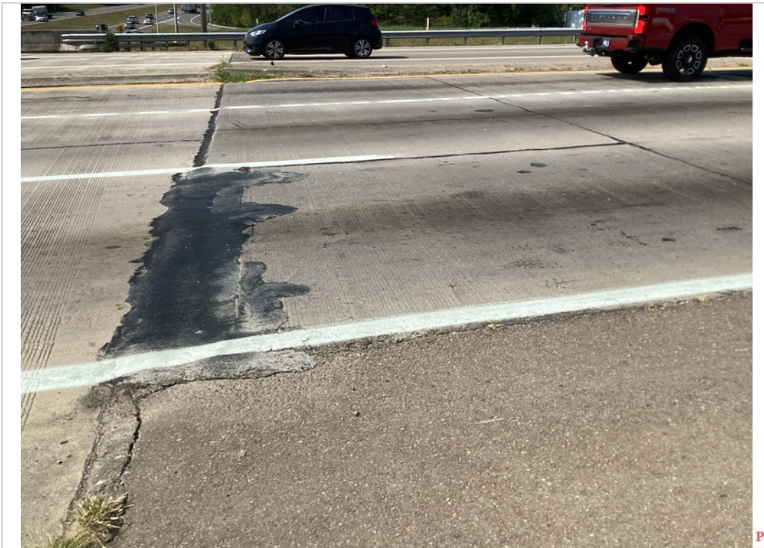
Approach 1 slab left lane - patched area
