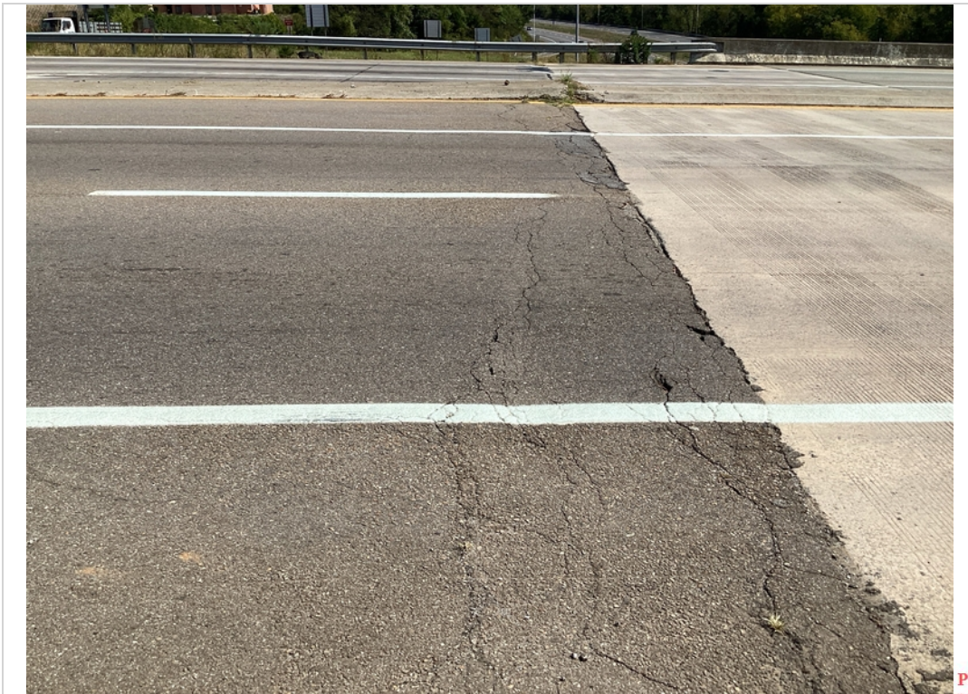
Approach 1 right lane wearing surface - patches, cracks to 1/8", areas ready to spall
