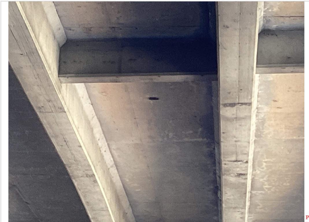
Bottom deck span 3 between beams D/E - Popout
