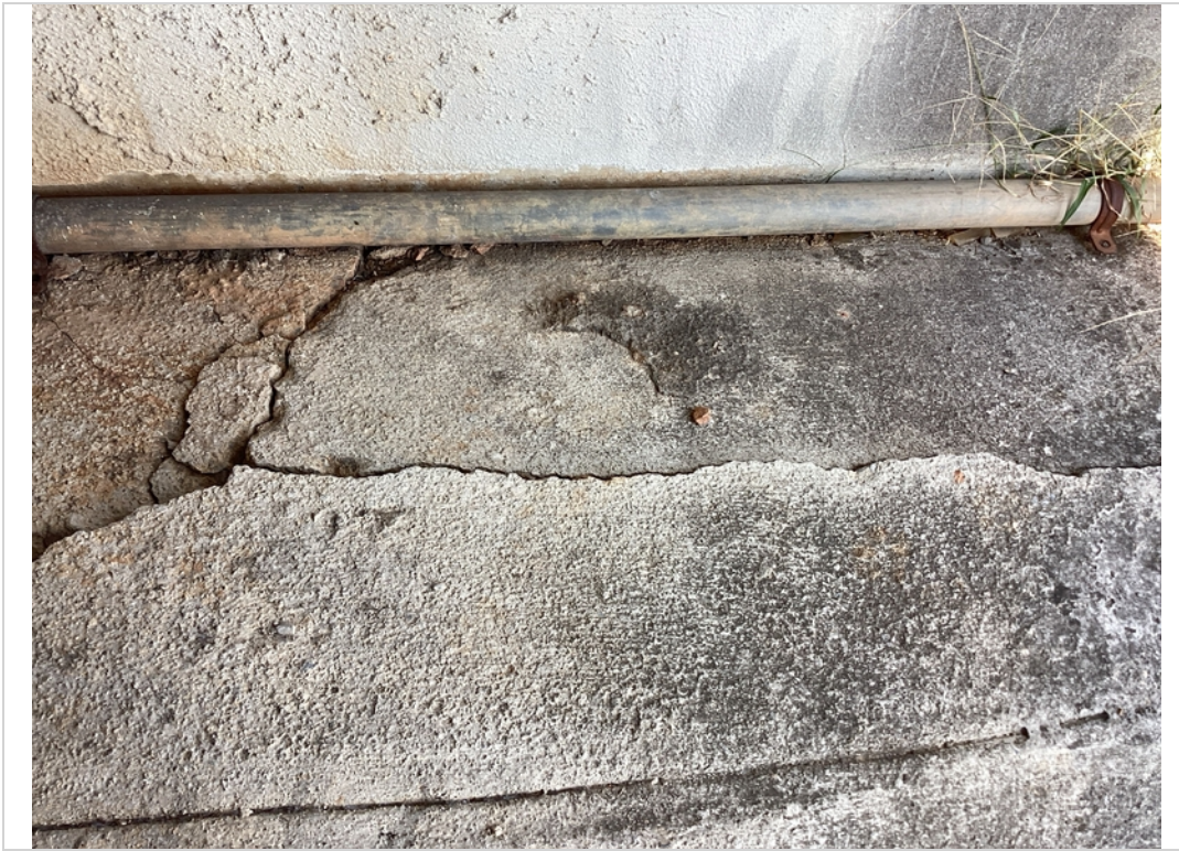
Abutment 1 left - concrete slope - Cracking up to 1/4"
