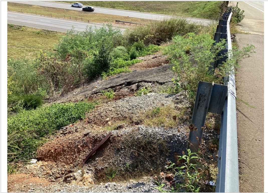
Approach 1 left embankment - erosion ditches, some with asphalt added
