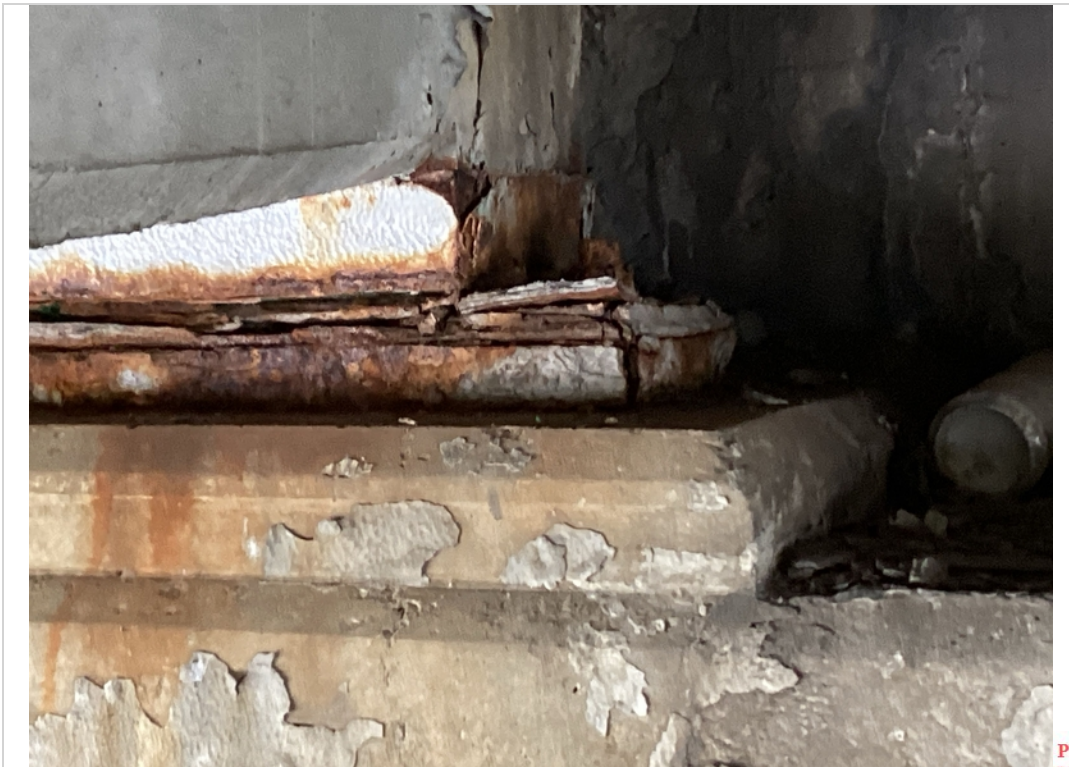
Abutment 1 Bearing I - Heavy corrosion and flaking
