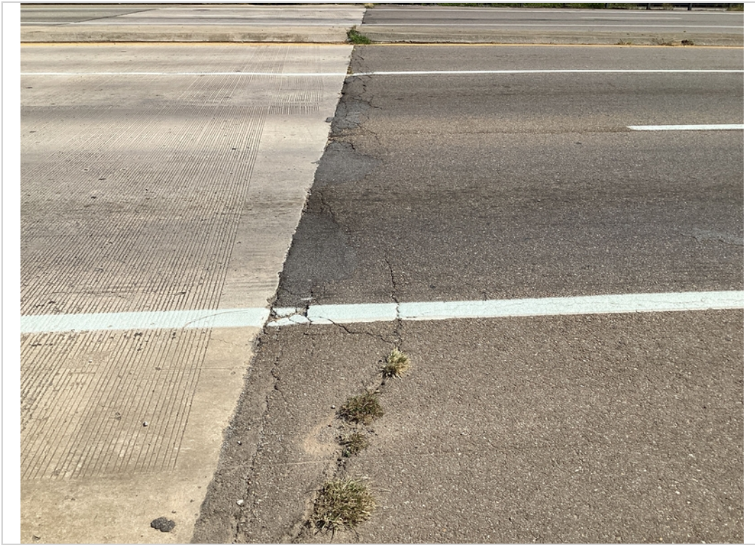
Approach 2 right lane wearing surface - patches, cracks to 1/8", areas ready to spall
