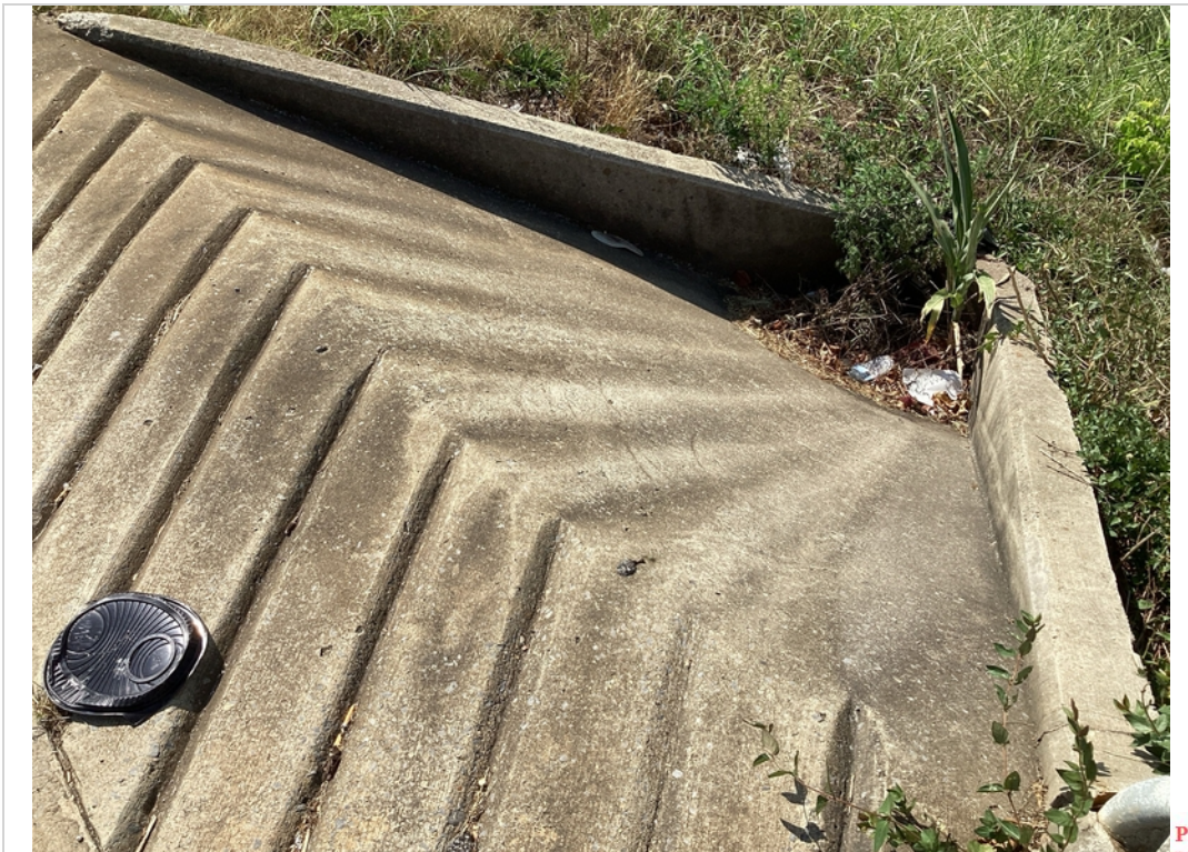
Approach 2 right drain - plugged
