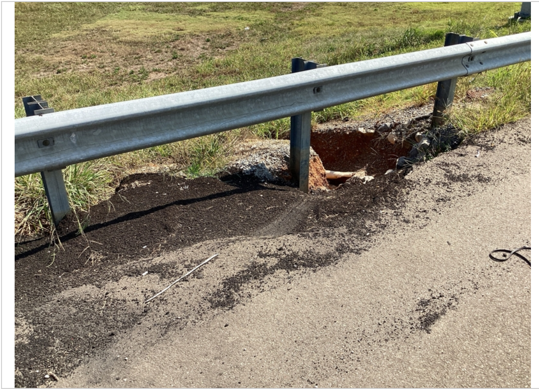
Approach 2 left embankment - erosion ditches with asphalt patch
