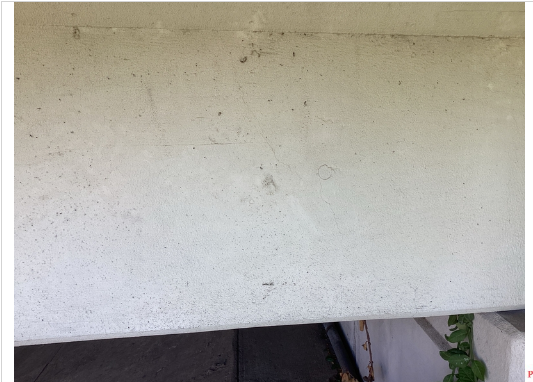
Span 4 Beam L right at abutment 2 - Diagonal hairline crack (Typical beam A left & beam L right abutment 1)
