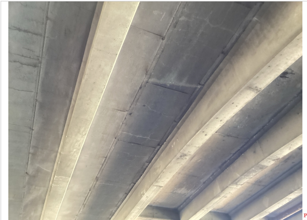
Span 2 bottom deck between beams E & F - Hairline cracks with leaching (typical)
