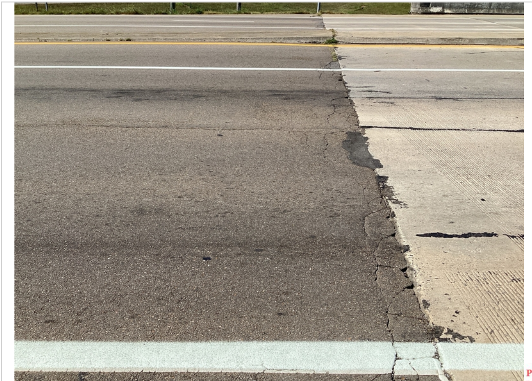
Approach 2 left lane wearing surface - patches, cracks to 1/8", areas ready to spall
