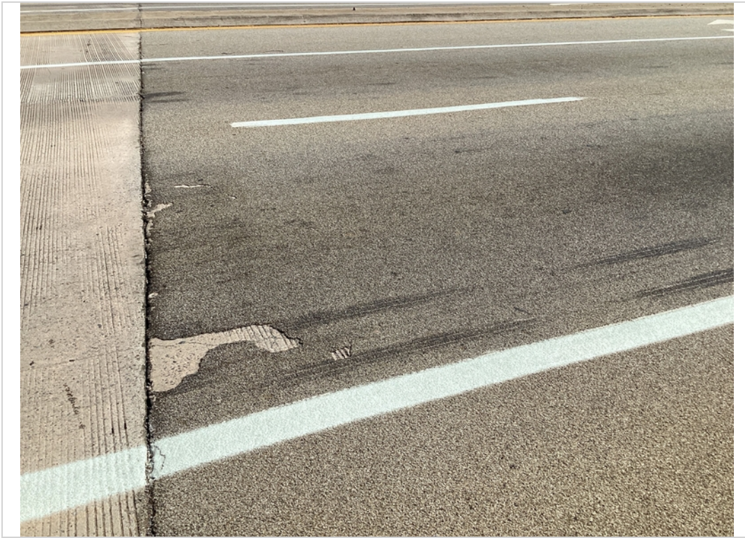
Deck 1 right lane - epoxy wearing surface scaled off
