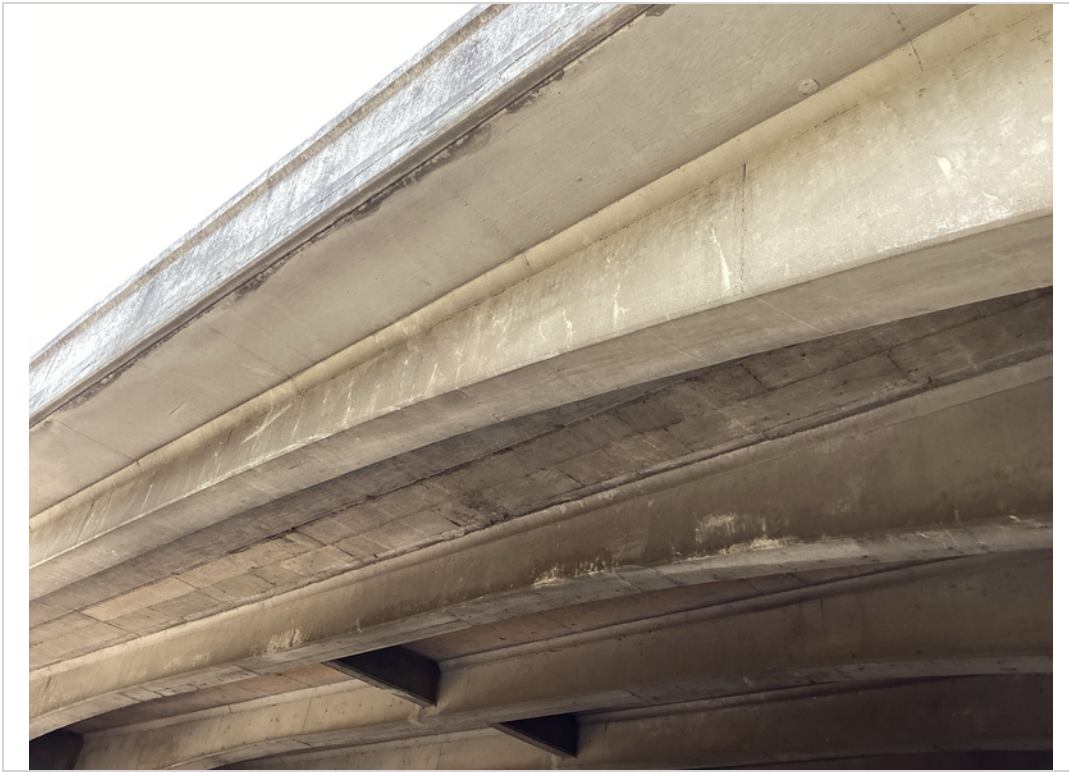
Span 2 beam L - Hairline cracks with leaching (typical )
