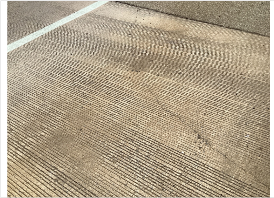
Approach 1 slab right lane - hairline crack
