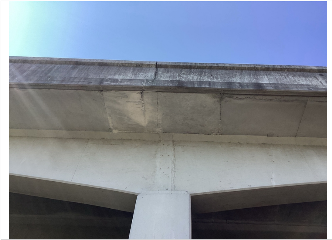
Bent 2 left overhang - Hairline cracks with leaching (typical )
