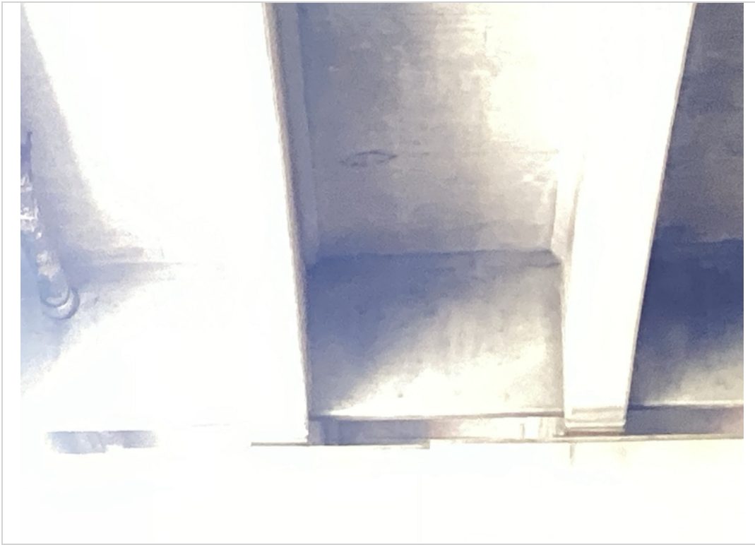
Bottom deck span 2 between beams C/D - In place spall (1' diameter)
